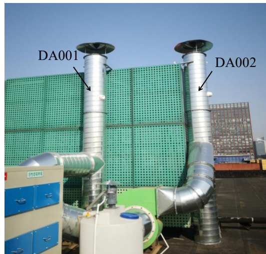
废气排气筒及出口监测孔
